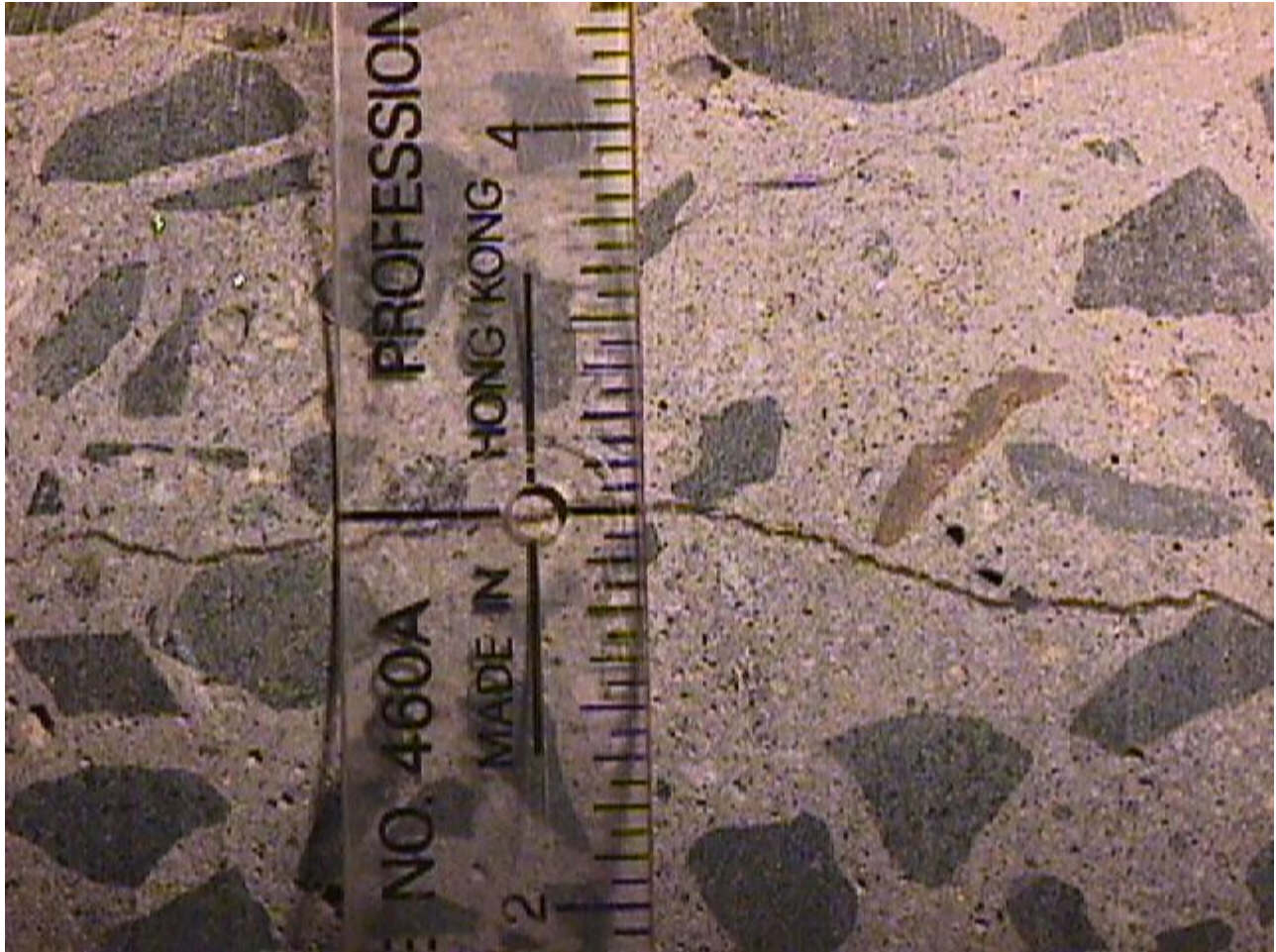
Penetration at 12"(305mm) deep
